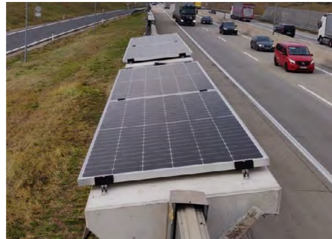
First test sections of the innovative power-generation solution
